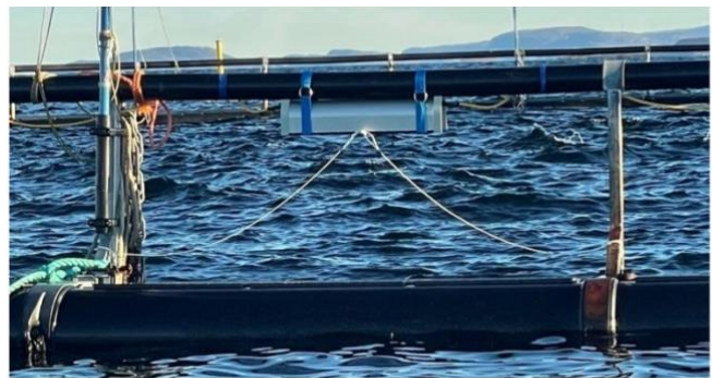
Figure 6. PDC mounted on handrail with secondary fuse.
