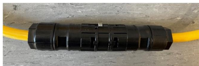
Figure 8. Connection of lamps to PDC
