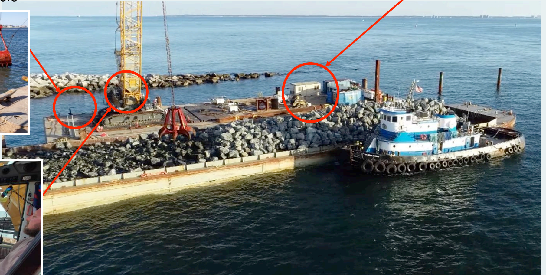
Remote access point
